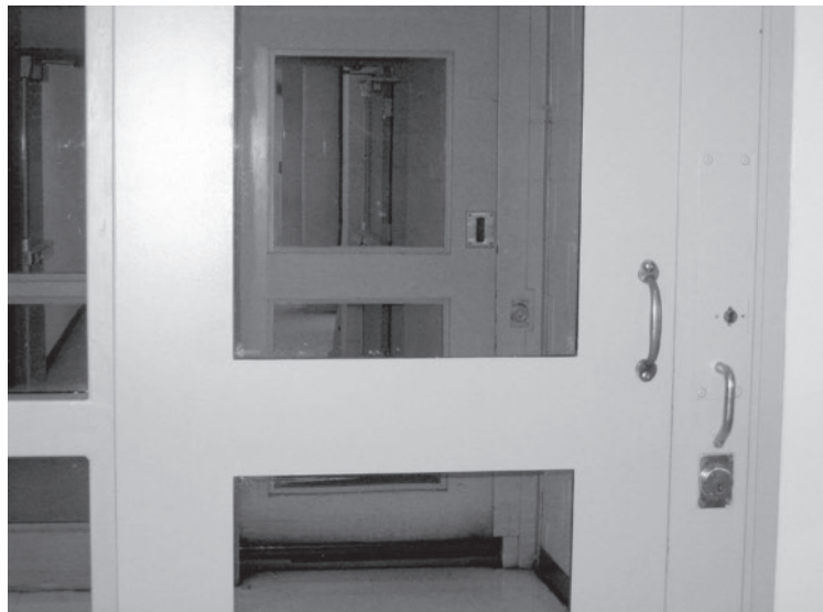
Figure 4-1 Doors that allow one section of passage to be closed before opening another section
